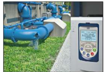
A WEG VSD detecting low pressure indicating leakage in a pipeline.
